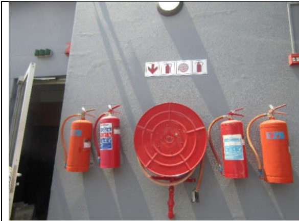
Image 1: some of the fire extinguishers and a hose pipe on site.
