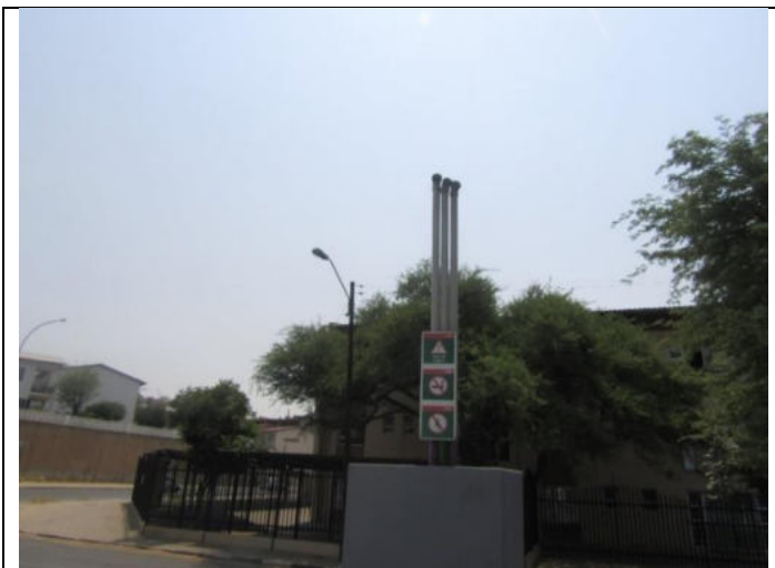
Image 1: Vent pipes have been installed on site (3m) to release vapors above the immediate atmosphere to enhance pollution attenuation.
