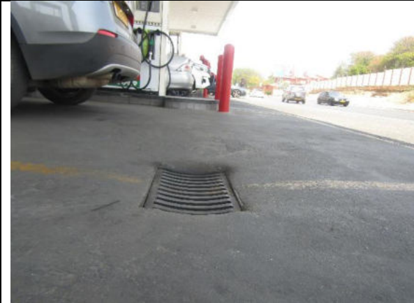
Image 1: Oil and water interceptor at filler points to collect wastewater and oils from the forecourt to the water and oil separator pits
