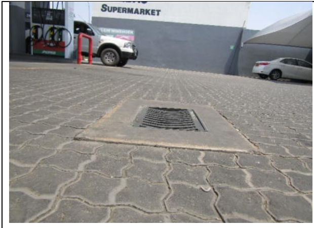
Image 1: Oil and water interceptor at fuel dispensing points to collect wastewater and oils from the forecourt to the water and oil separator pits
