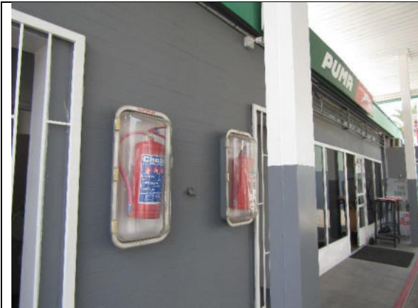
Image 1: some of the fire extinguishers on site.
