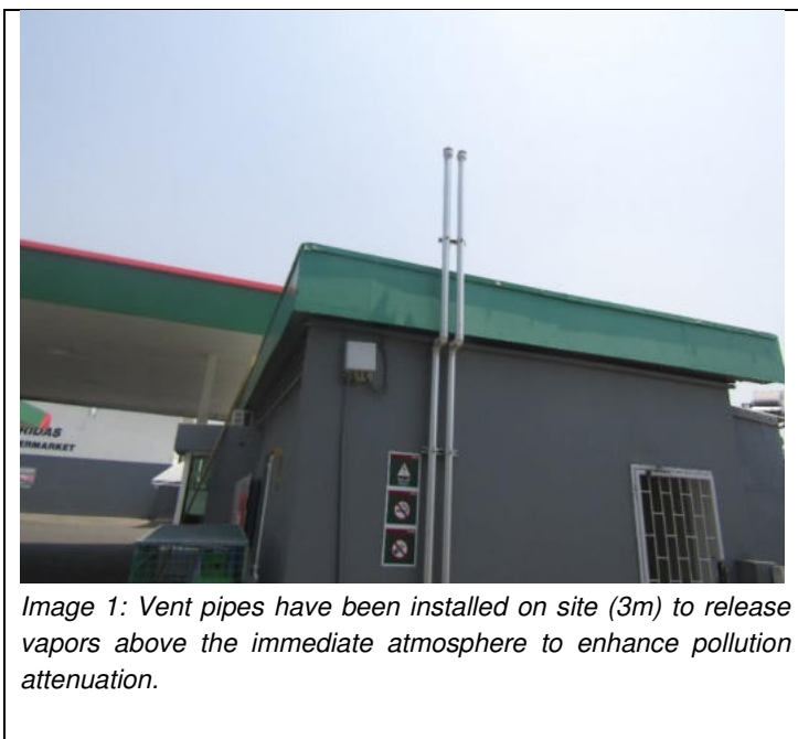
Figure 3: hydrocarbon vapours and odours pollution control measures currently on site
