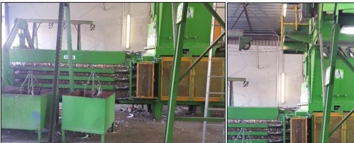
Figure 12: Compressing and baling equipment
