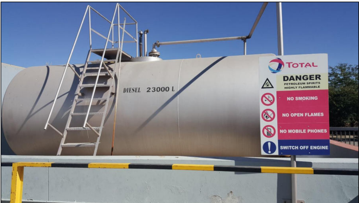
Figure 16: Fuel Storage Tank
