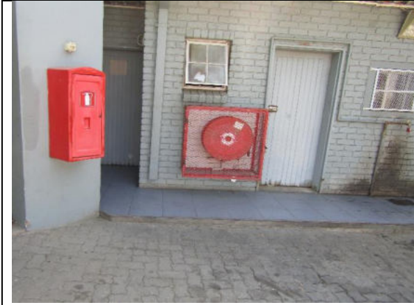
Image 1: One of the fire extinguishers and a hose pipe on site.
