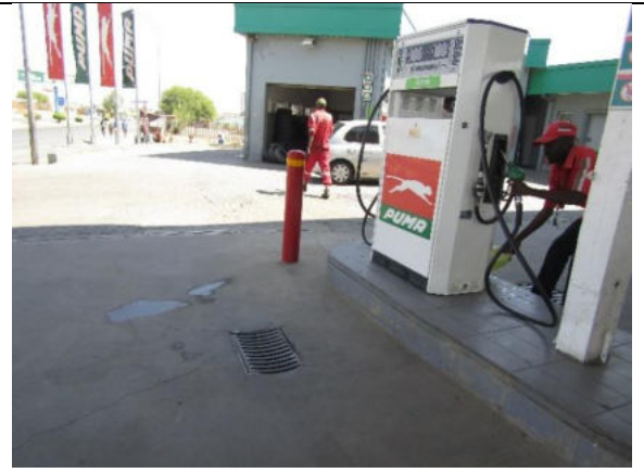
Image 2: A concrete slab at dispensing points and around tanks filler area for oil spill containment.
