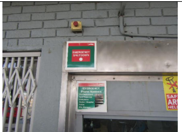
Image 4: emergency shutdown alarm.
