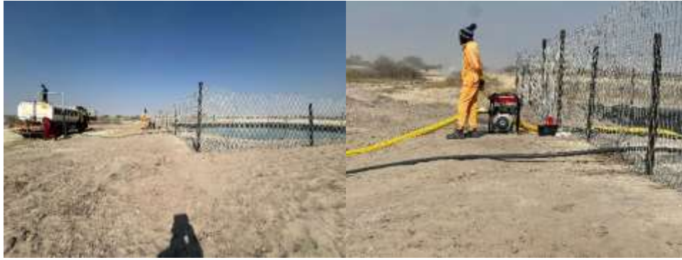
Figure 2-11: The water holding dam between Ondjamba and Engoyi
