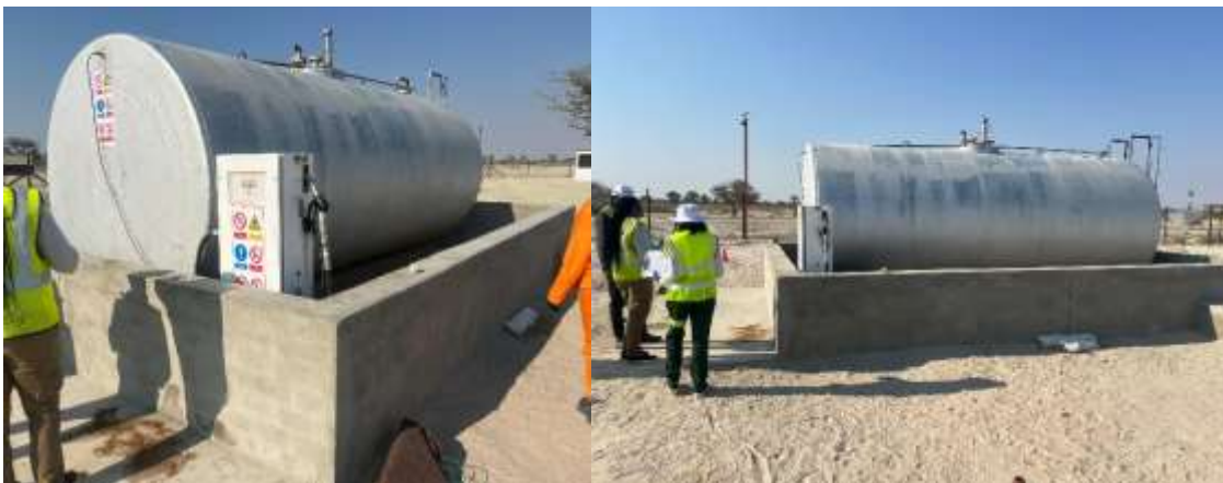
Figure 2-12: The diesel (fuel) tank within the contractors' campsite near Engoyi Settlement
