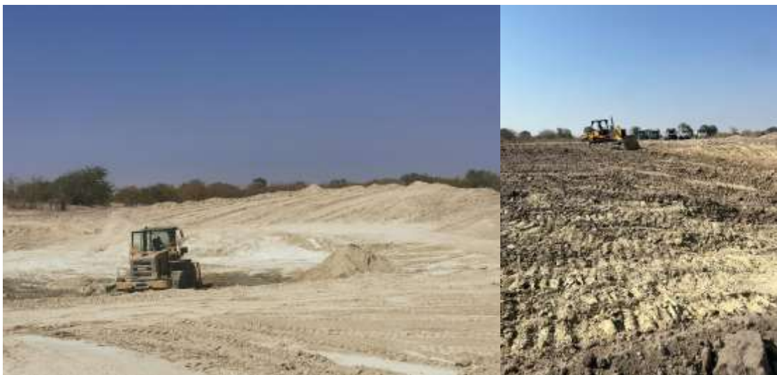
Figure 2-10: Excavator at BP 15 RHS site as well as excavator and 5 dump trucks at BP6 site
