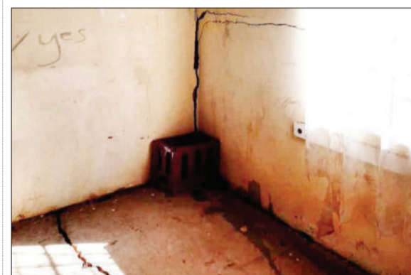
Dilapidated... The Epukiro Kindergarten in Omaueozonjanda is in a perilous state.
