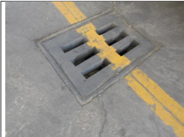
Image 1: Oil and water interceptor to collect wastewater and oils from the forecourt to the water and oil separator pits
