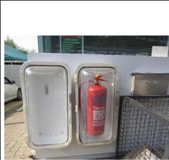
Image 1: one of the fire extinguishers on site.
