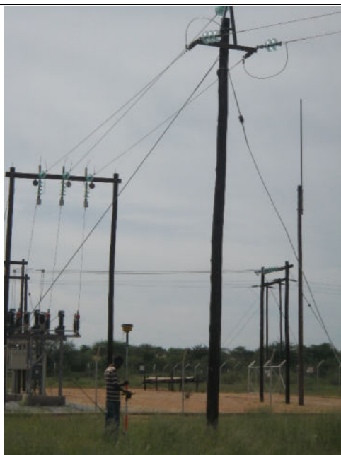
Photo 5.5 – View of Electrical Substation
