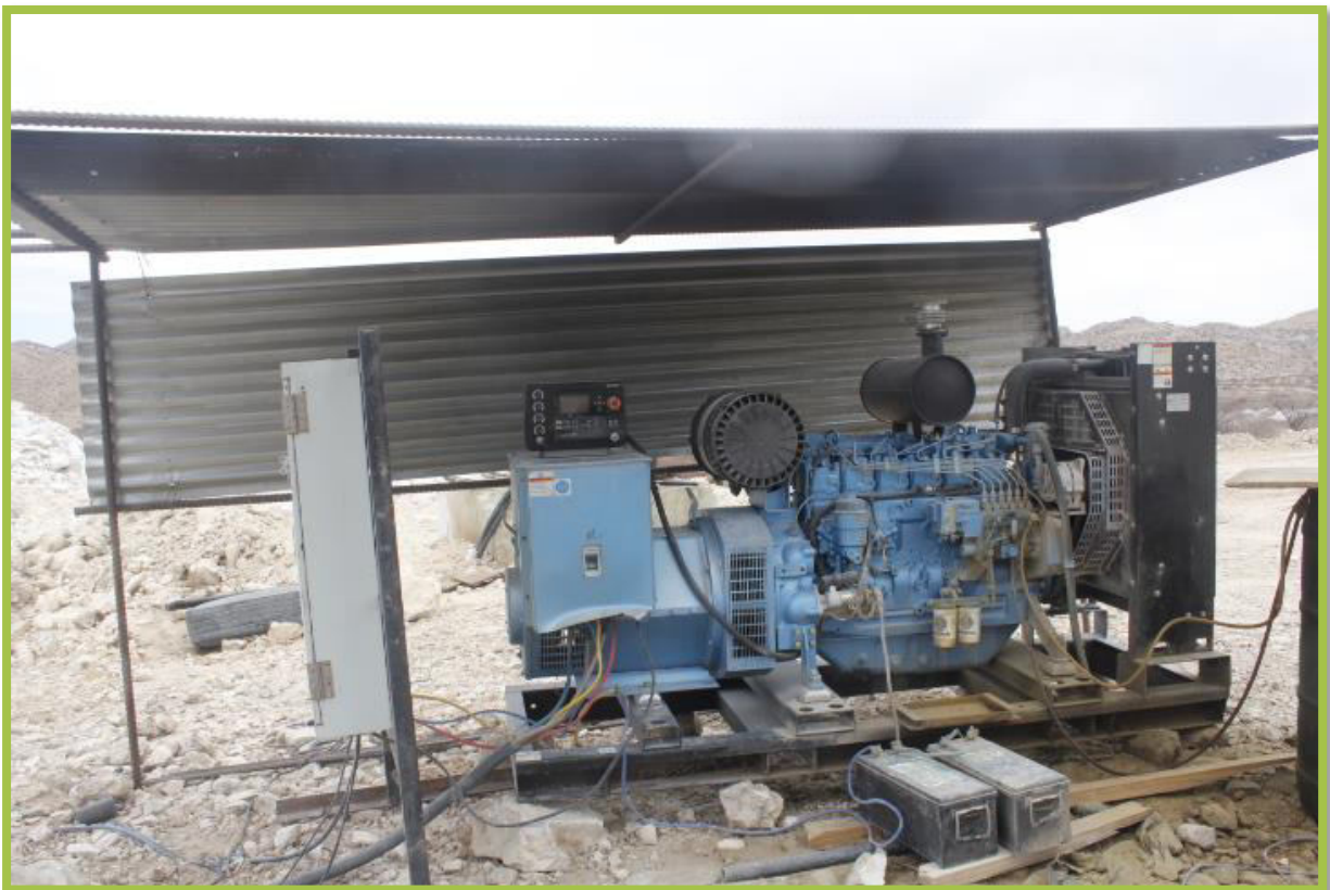
Figure 4: A 275 KV generator that will supply power to at the site.
