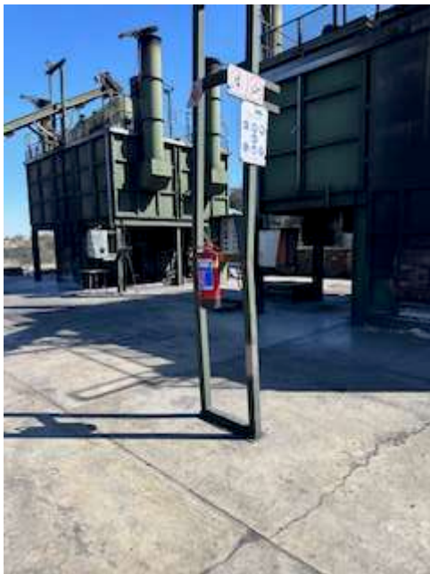
Figure 6 - Fire-extinguishing equipment in dedicated work areas (provided by the Proponent)
