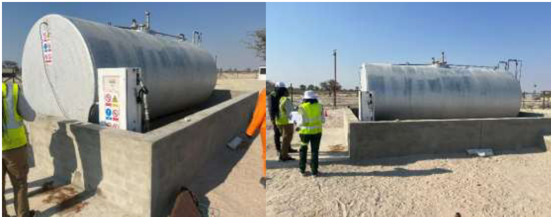
Figure 2-1: The diesel (fuel) tank within the contractors' campsite near Engoyi Settlement
