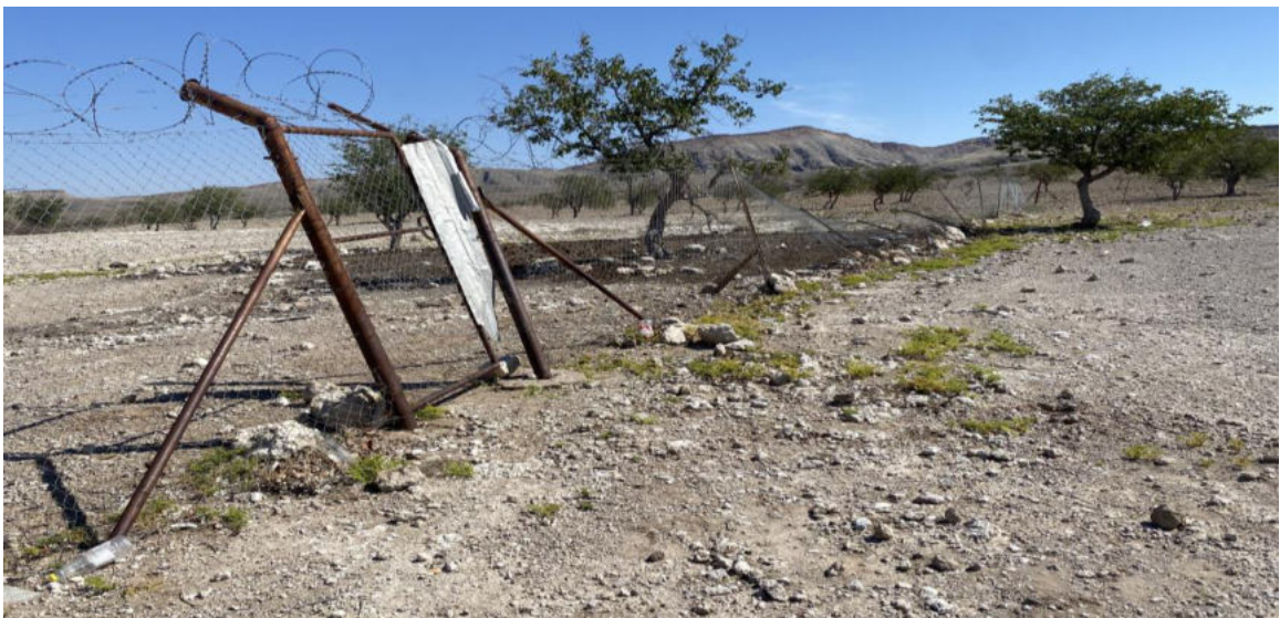
Figure 2-3: The perimeter fence surrounding Sesfontein APU; some parts of the fence are falling apart
