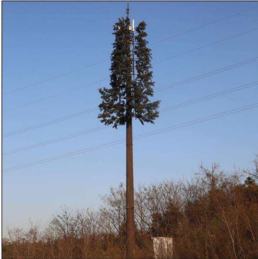
Figure 2: Example of a camouflaged tree telecommunication tower
