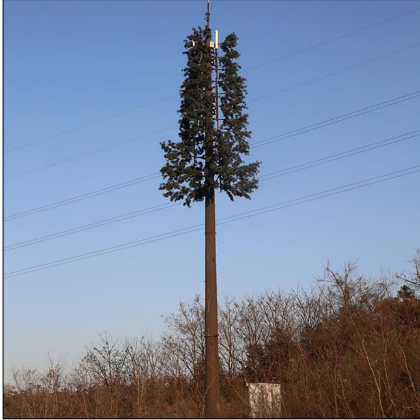
Figure 3: Typical example of a camouflaged telecommunication tower structure
