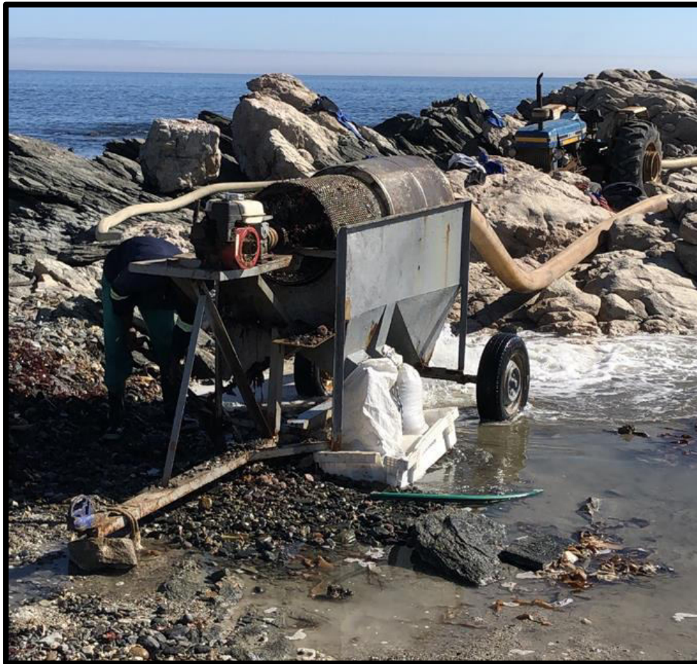
Figure 6: Picture showing a sediment delivery pipe running from the tractor to the trommel screen ( Source: Anonymous, n.d. ).
