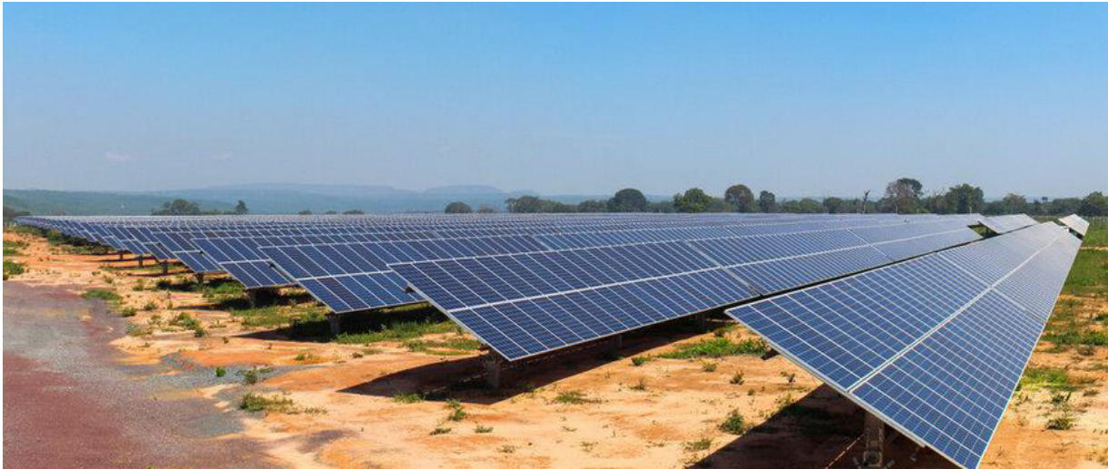
Figure 2: Illustrate the typical installation of solar panel filed, similar to which DanAon Energy envisage to install
