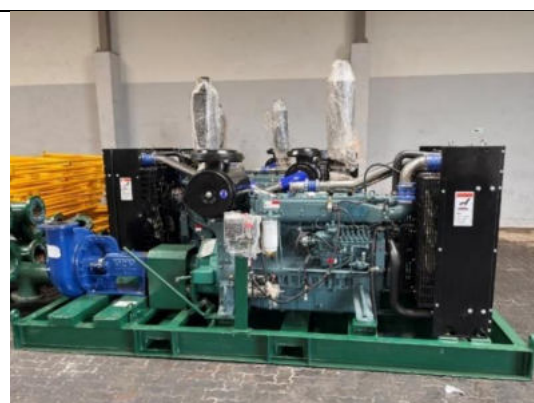
Photo 4-4 Diesel driven centrifugal pump
