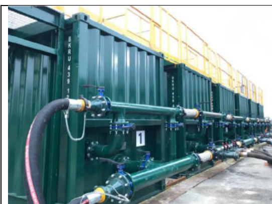
Photo 4-1 Drilling and completion fluid storage tanks
