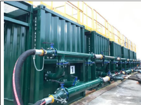
Photo 4-5 Drilling and completion fluid storage tanks
