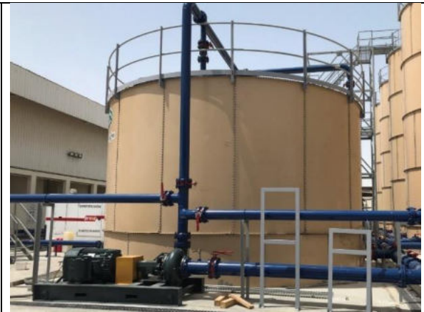
Photo 4-6 Fluid mixing tank
