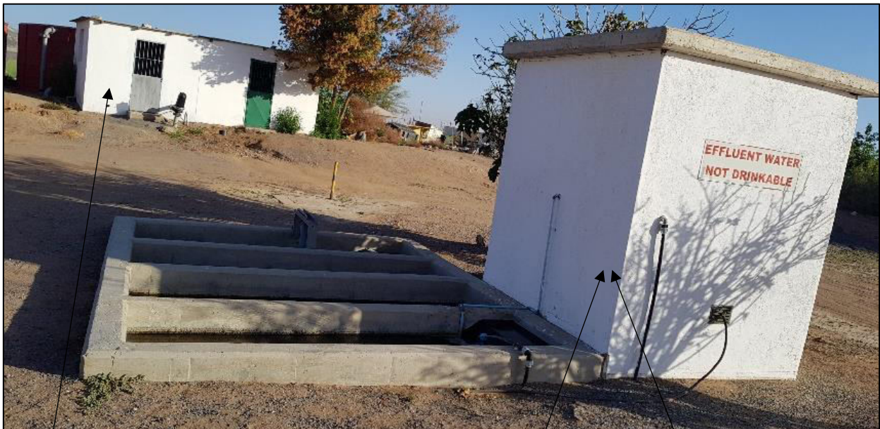
Figure 9: Chlorine contact room & Pump station room
