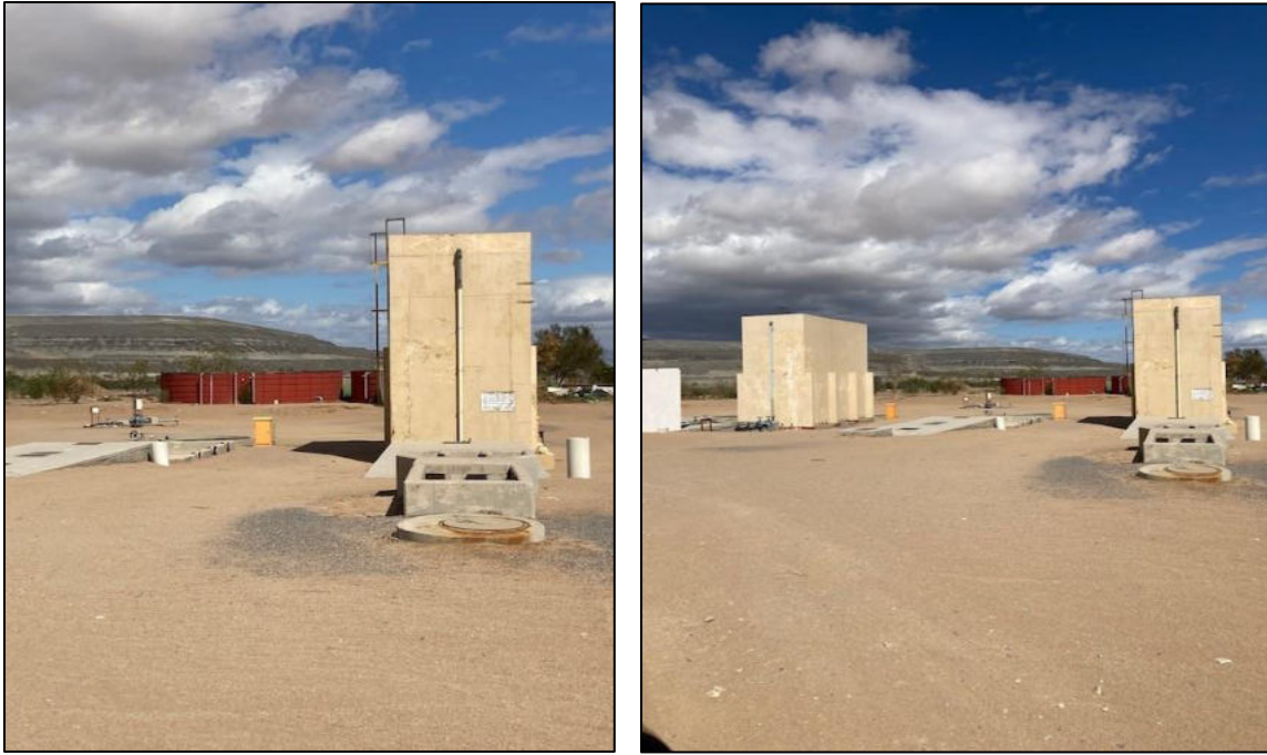
Figure 11: Sewage collection point (to sort out any solid wastes) and the Trickle Filter Towers (where sewage is broken down into smaller organisms)
