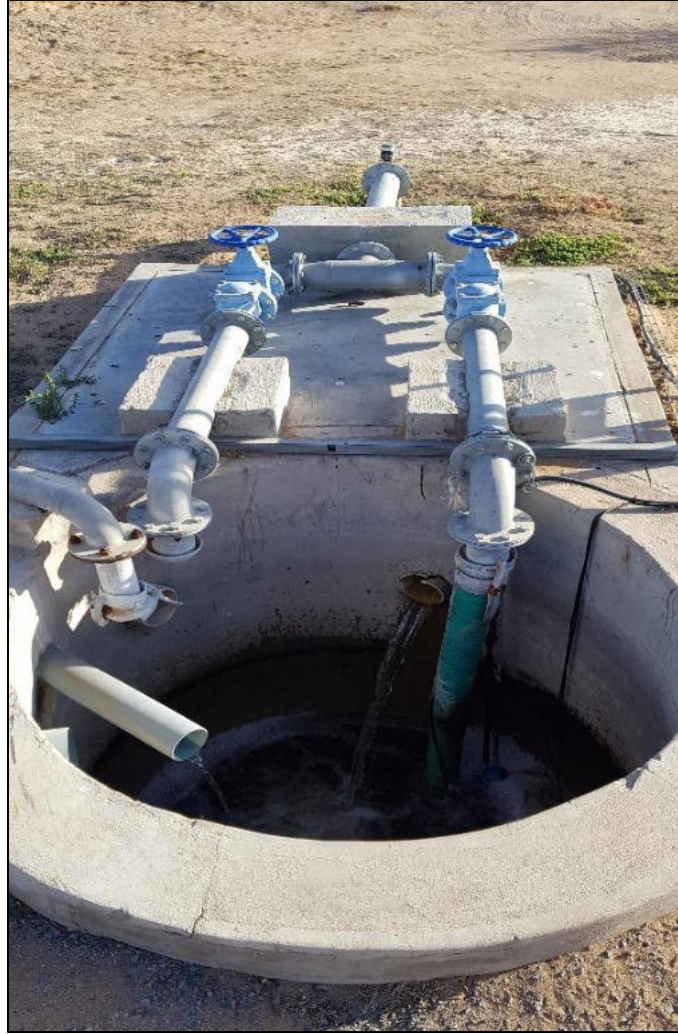
Figure 6: Treated water collection point
