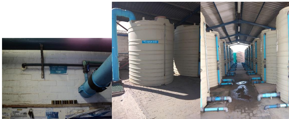
Plate 11: Transfer pumping of treated and disinfected seawater to 16 storage tanks of 10,000 liters.
