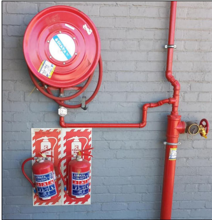
Figure 14: One of the fire extinguishers on site
