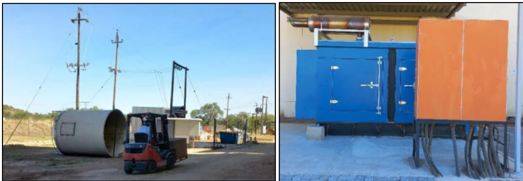
Figure 11: Electricity source on site and back-up generator
