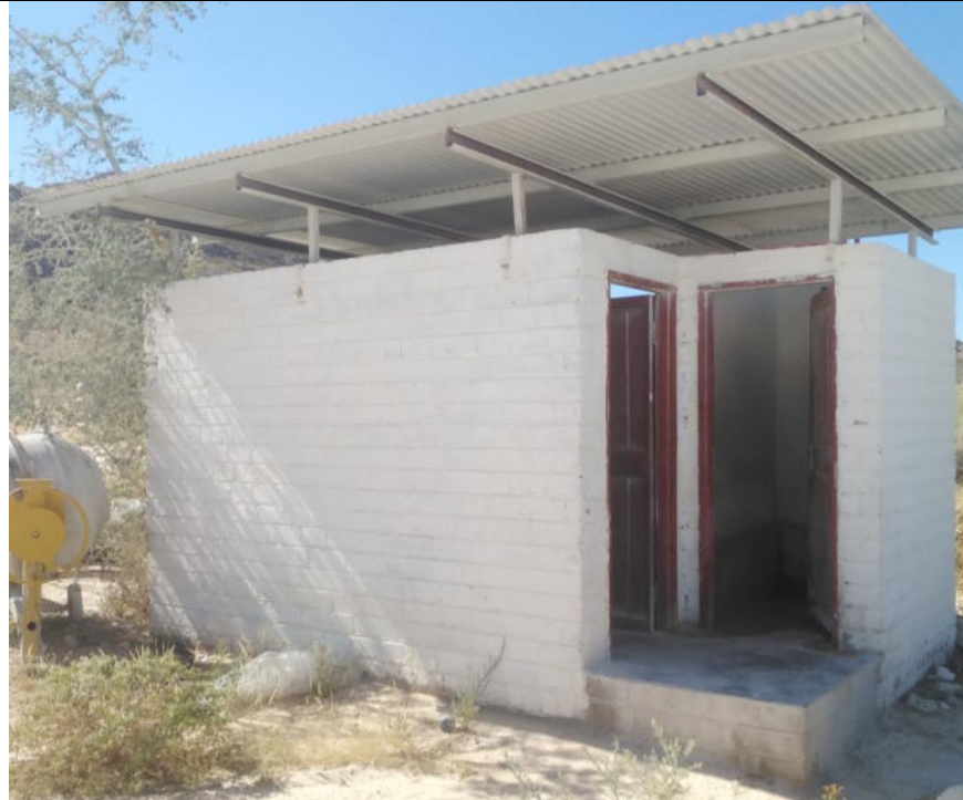
On-site Ablution Facilities for the staff at the mine
