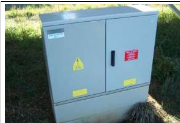
Photo 5-3 Typical array junction box
