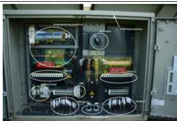
Photo 5-4 Typical array junction box
