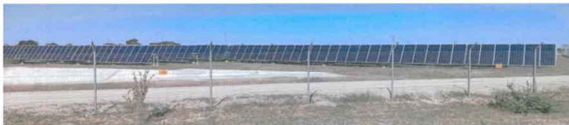
Figure 3: The operational NCF Energy (Pty) LTD IPP 5 MW Solar PV Power Plant in Engoyi Village, Okatope (HEEC,2022)
