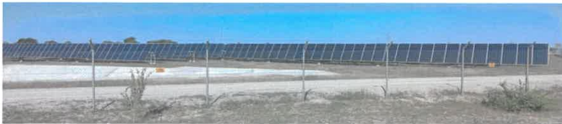
Figure 3: The operational Tandii Investment (Pty) LTD 5 MW Solar PV Power Plant in Engoyi Village, Okatope (HEEC,2022)
