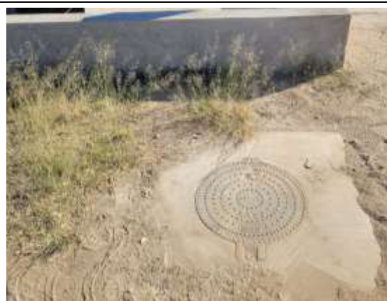
Photo 4-4 Oil water separator
