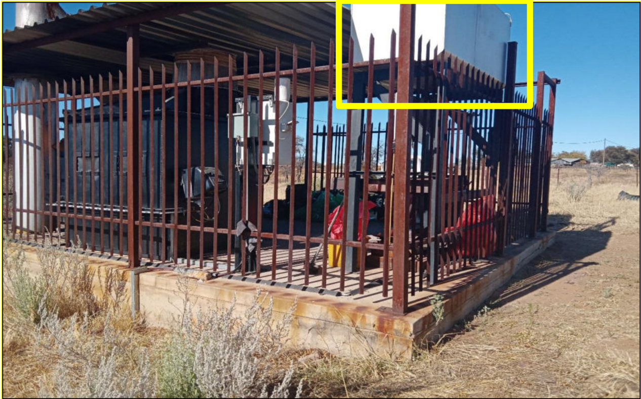
Figure 6: Shows the safely mounted 1000 litres diesel tank (yellow outline)
