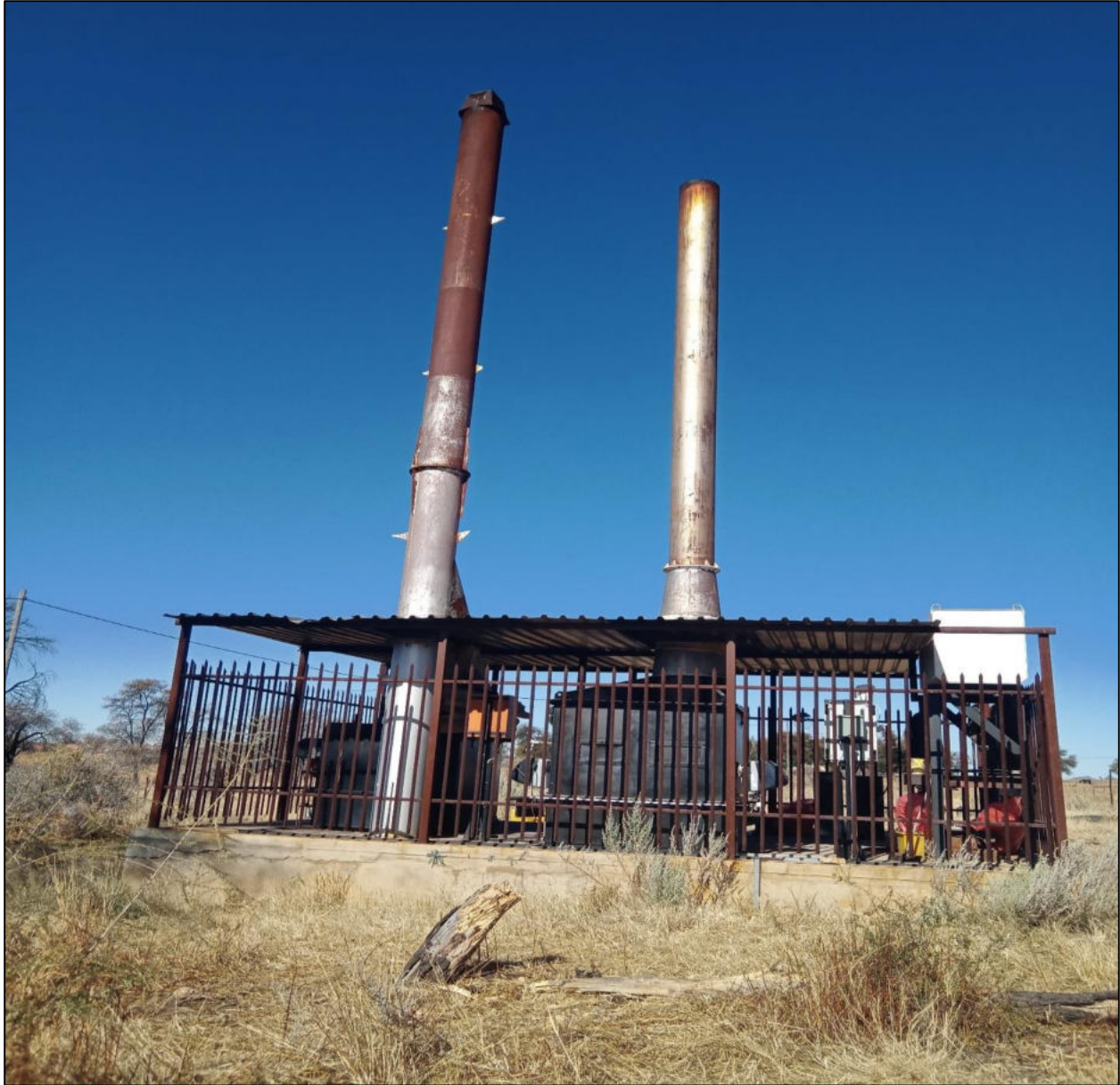
Figure 3: Shows the rear (back) side of the incinerators.
