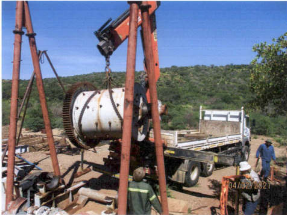
PHOTO 2: The old ball mill being loaded by the crane lorry, for transport to Onganja Mine. The gantry in the foreground was also dismantled and removed.
