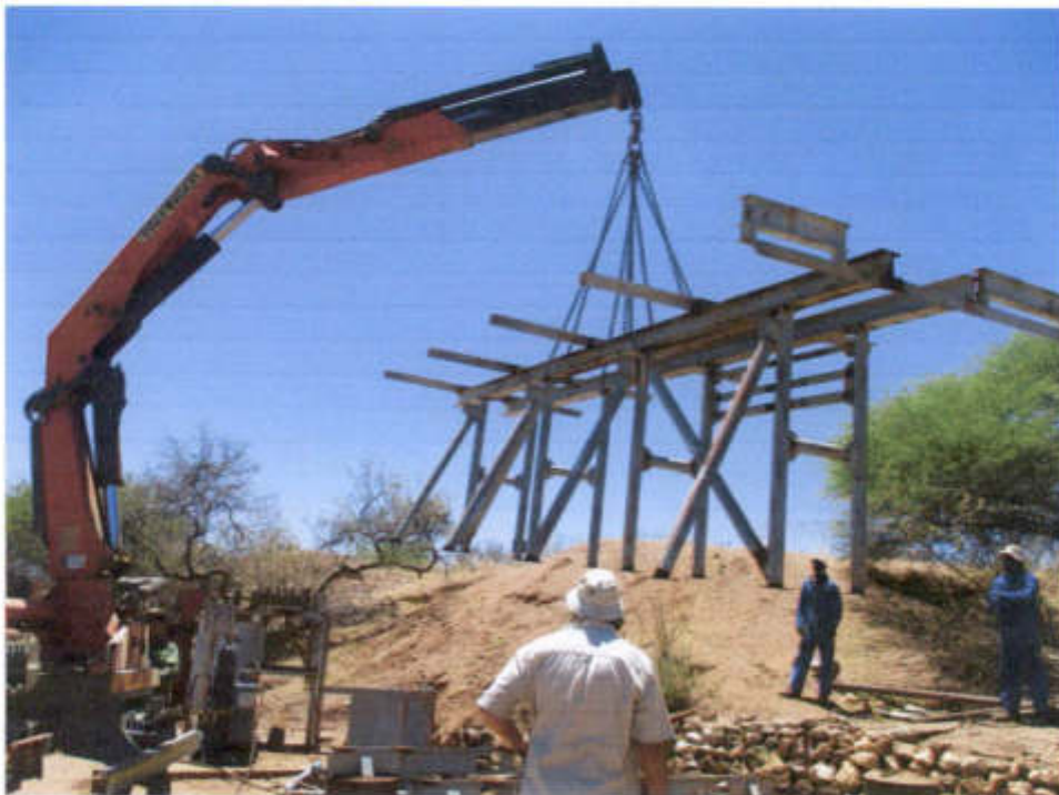
PHOTO 3: View of the lorry crane lifting the flotation cells framework off its base, while the loading operation was underway. The cells had been already loaded and removed to Onganja Mine.
