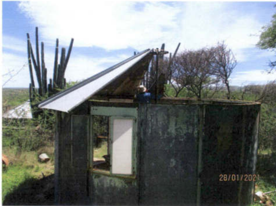
PHOTO 4: As part of the rehabilitation programme, the derelict workers' accommodation rondavels are being dismantled and removed. The photo shows the dismantling work in progress, the roof being first removed.
