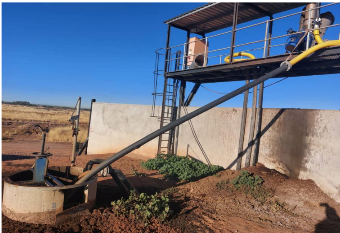
Figure 7: Picture showing the solid separator or screw press (Source: Miss Gloudi de Beer, August 2022).
