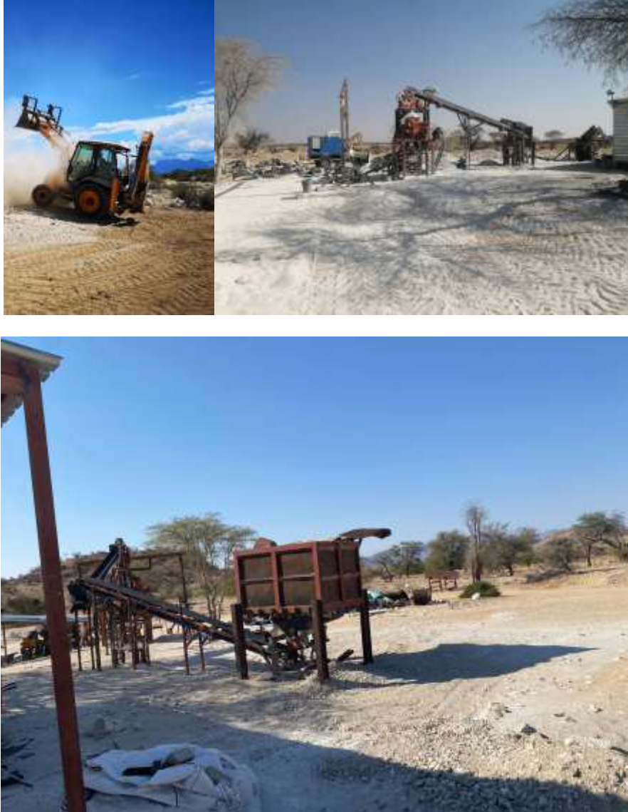
Figure 2-3: Some of the site machinery and equipment (the TLB and conveyor belt system)
