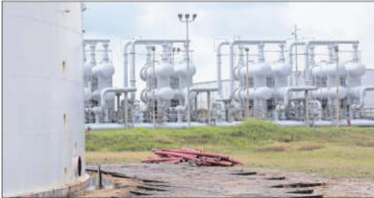
An oil storage tank and crude oil pipeline equipment is seen during a tour by the Department of Energy at the Strategic Petroleum Reserve in Freeport. PHOTO REUTERS
