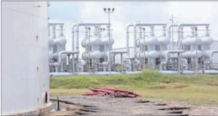
An oil storage tank and crude oil pipeline equipment is seen during a tour by the Department of Energy at the Strategic Petroleum Reserve in Freeport. PHOTO REUTERS
