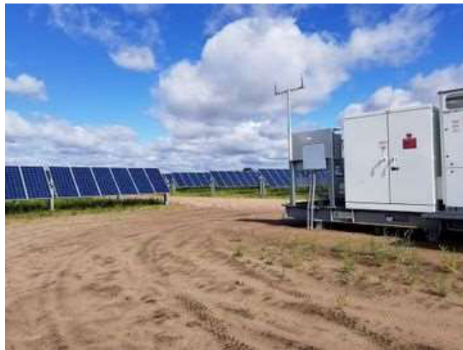
Figure 6: A photovoltaic system comprised of a solar panel array, inverter and other electrical hardware (Source: https://energyeducation.ca/encyclopedia/Photovoltaic_system ).
