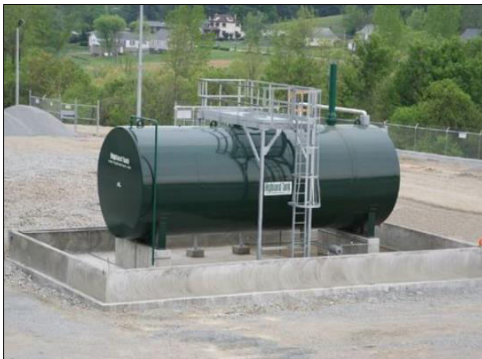
Figure 2-2: An example of a fixed fuel storage tank, installed on paved ground to minimise the risk of pollution.
