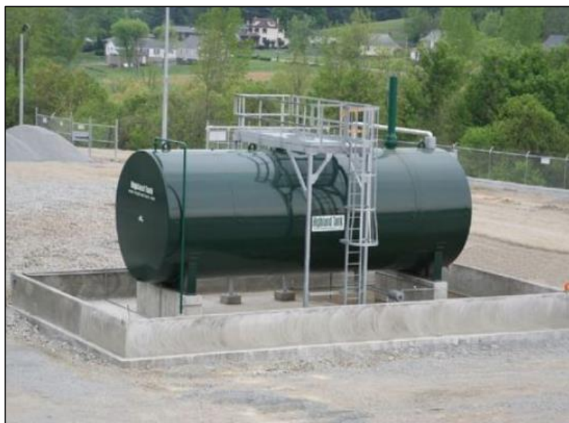
Figure 2-1: An example of a fixed fuel storage tank, installed on paved ground to minimise the risk of pollution.
