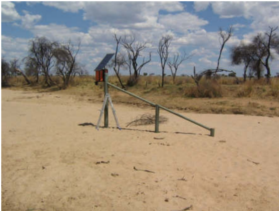
FIGURE 9-3: BLACK NOSSOB SITE (WW202120) DATA LOGGERS.
