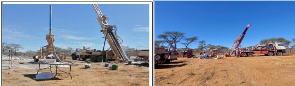
Figure 2-4: A drill rig on an EPL in the Omaheke Region (Resilient Environmental Solutions, 2022)
