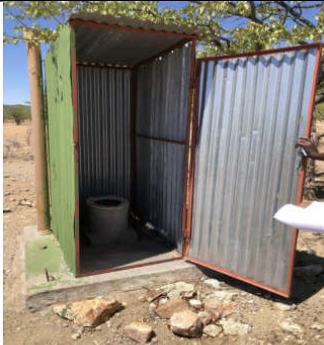
Fig3. Currently being used, a pit latrine toiled sited about 80m from the construction Camp
