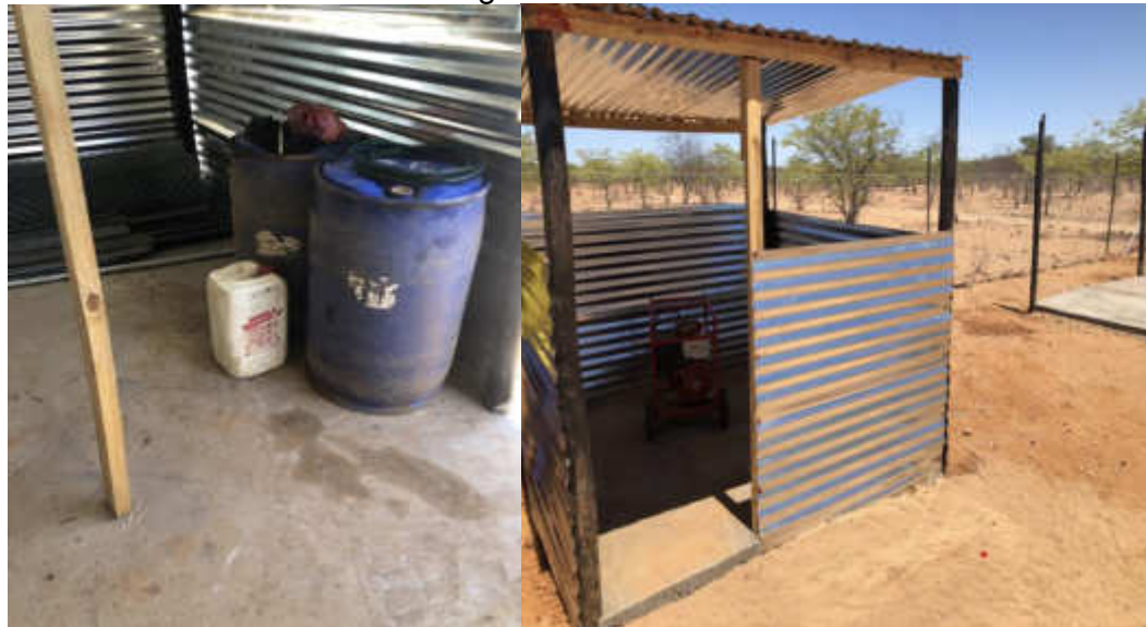
Fig4. Left is showing current storage of fuel in the contractor's storeroom posing risk to property and life. Right is showing recommended fuel containers and generator storage Facility.
