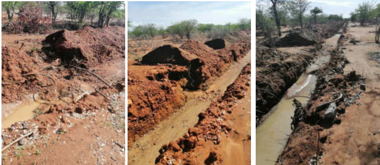
Fig1. Massive erosion that occurred on site, as evidenced by the Image further left and right, water was breaking through the overburden materials. Center image also highlights circumstances of trench walls collapsing.
