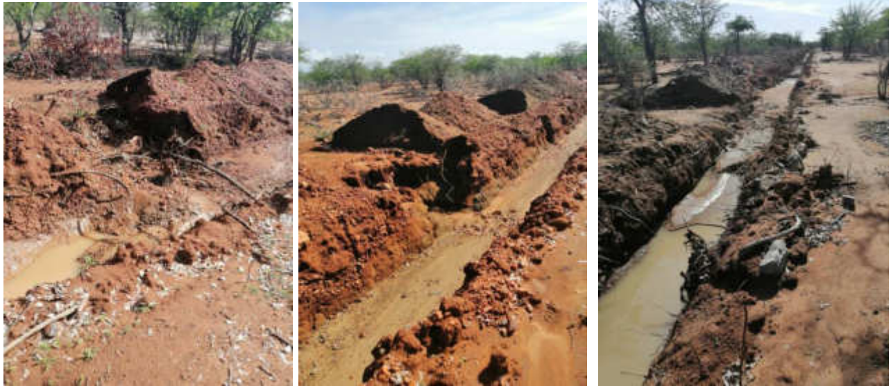
Fig1. Massive erosion that occurred on site, as evidenced by the Image further left and right, water was breaking through the overburden materials. Center image also highlights circumstances of trench walls collapsing.
