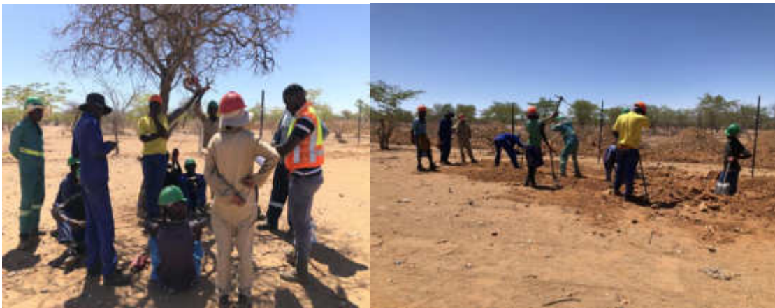
Fig5. Left is showing construction site Induction meeting conducted by the ECO and the Site Agent. Right is showing incomplete PPE worn by employees on site, necessitating need for PPE supply.
