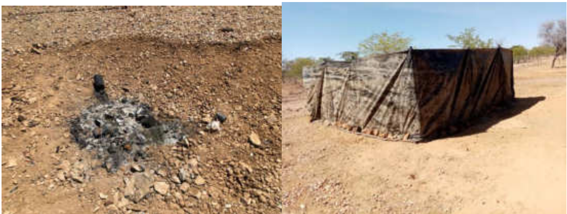
Fig6. Uncovered temporary waste storage site and waste burning was being done on site. Right is showing corrective action demarcating temporary waste storage site and covered with a net.
