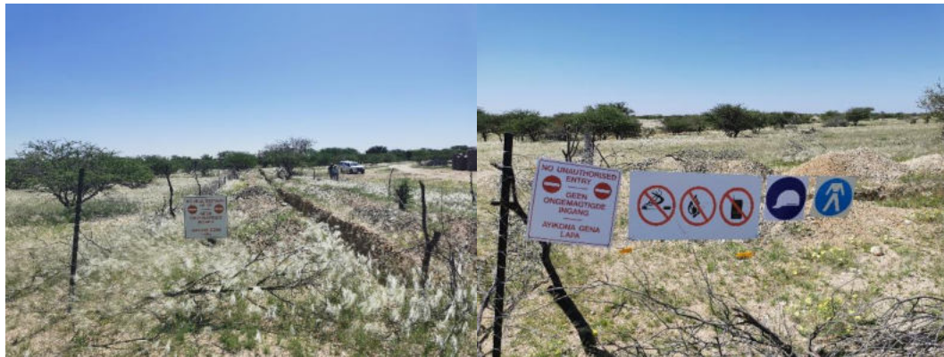
Figure 2-4: Fenced off exploration trenches awaiting backfilling upon completion of sampling (photos recently taken by Author at an ongoing precious metals exploration site visited by the Author in Erongo Region)
