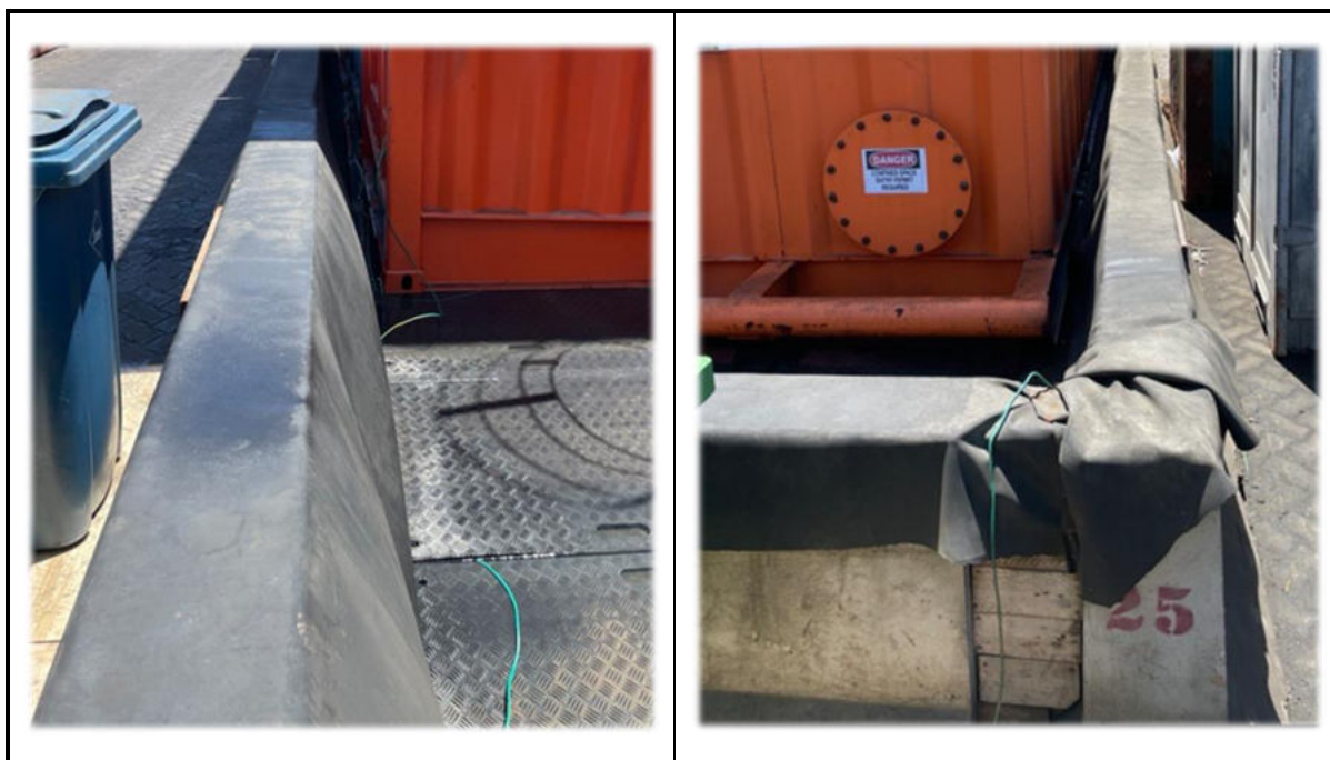
Photo 5: Moveable concrete bunding slabs
