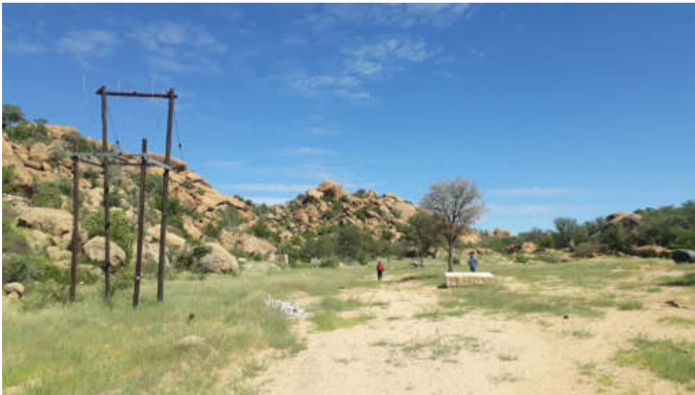
Figure 5: The electricity (power supply) lines in the project site
