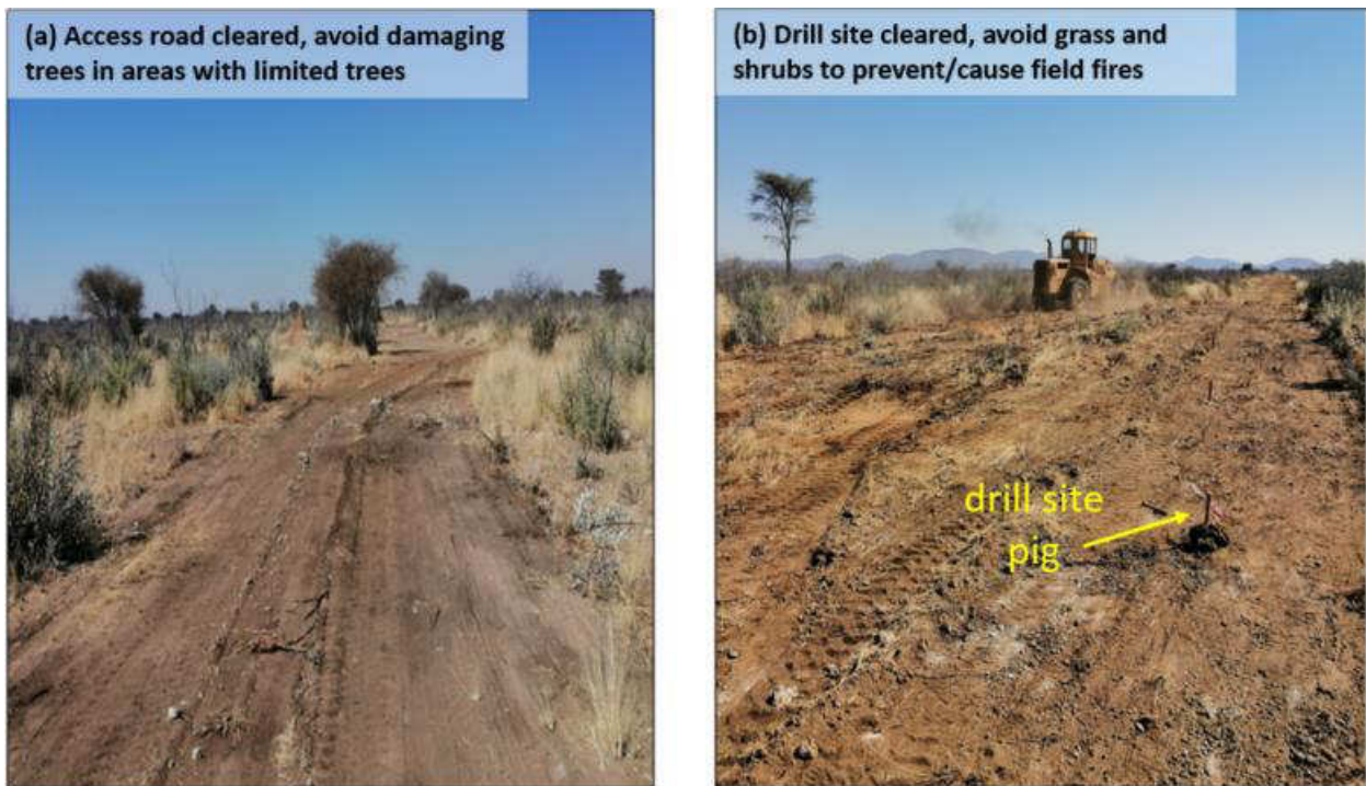
Figure 3 - Plates 1 (a): Access road cleared avoid damaging trees where limited, (b): Clearing drill site on the access road
