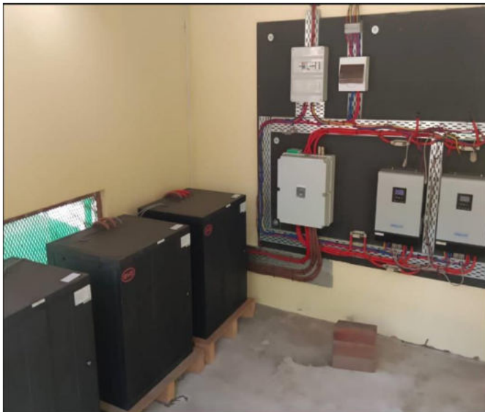
Figure 7: utility services available on-site
