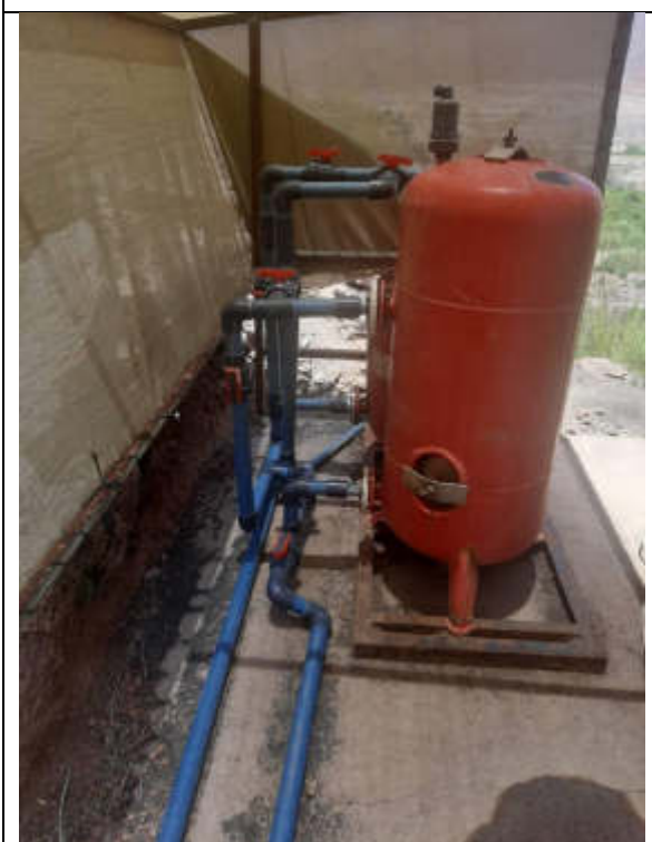
Photo 3 Sediment filter for main water tank
