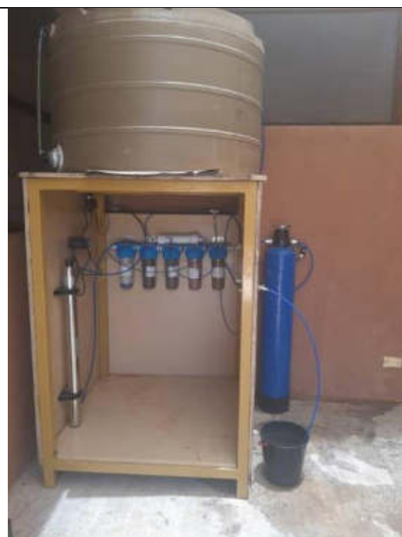
Photo 4 Drinking water filtration system
