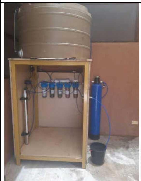
Photo 3 Drinking water filtration system
