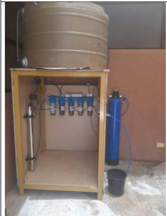
Photo 3 Drinking water filtration system
