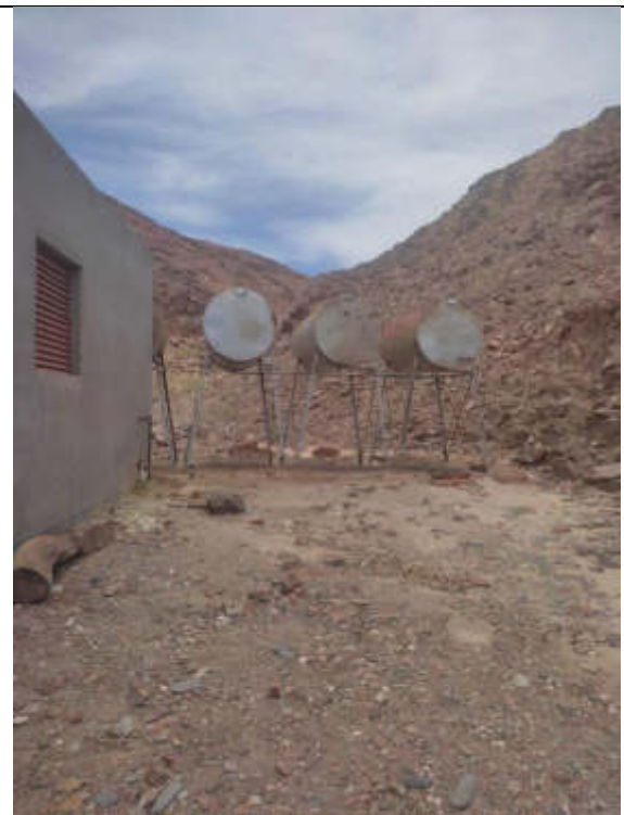
Photo 4 Consumer fuel installation
