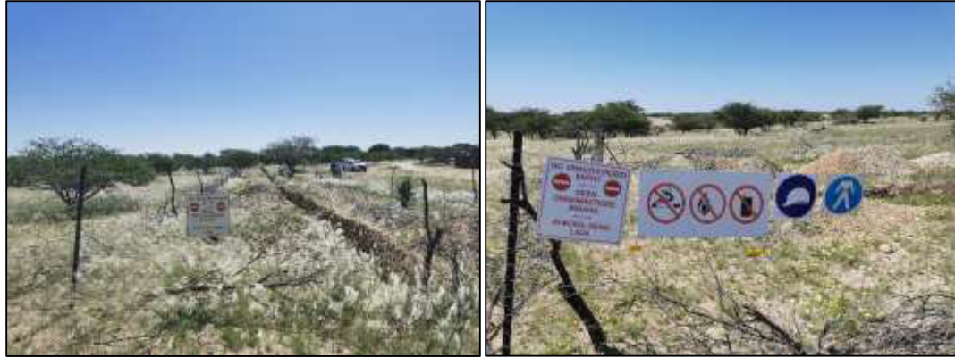
Figure 2-5: Fenced off exploration trenches awaiting backfilling upon completion of sampling (photos recently taken by Author at an active EPL visited by the Author)
