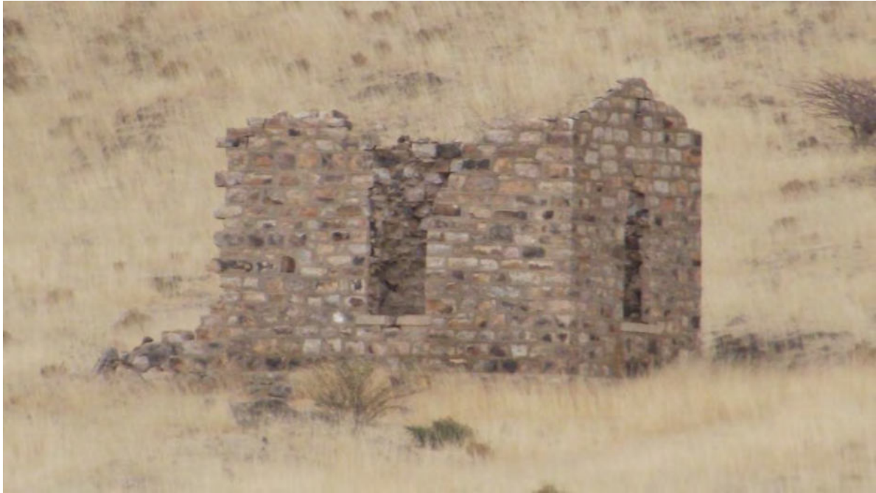
Figure 12; A ruined building structure (source: Authors 2022).
