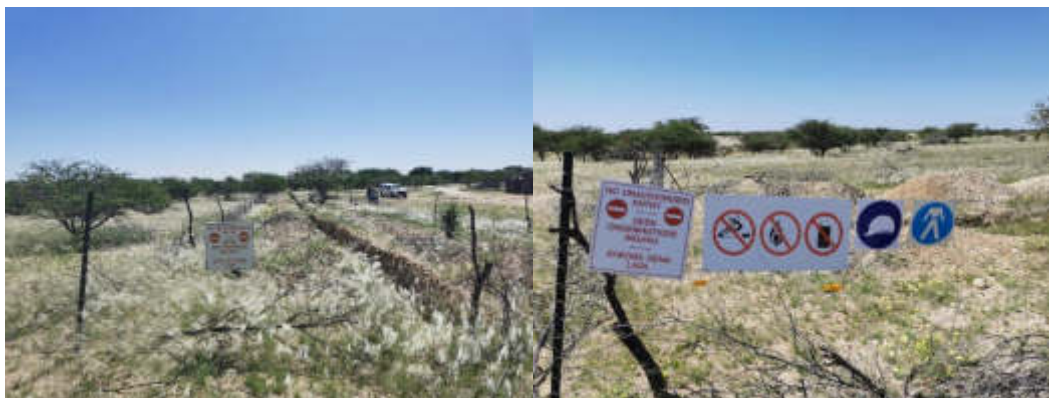
Figure 7: Fenced off exploration trenches awaiting backfilling upon completion of sampling (photos recently taken by Author at an ongoing precious metals exploration site visited by the Author in Erongo Region
