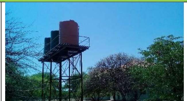
Figure 5: Water Storage Tanks
